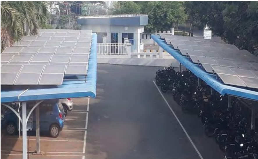
Onsite Roof solar plant in the parking areas
